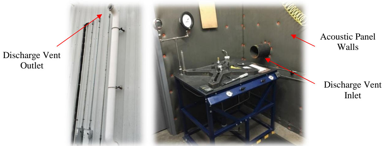
Figure 3: Typical Discharge Venting and Test Room Interior
